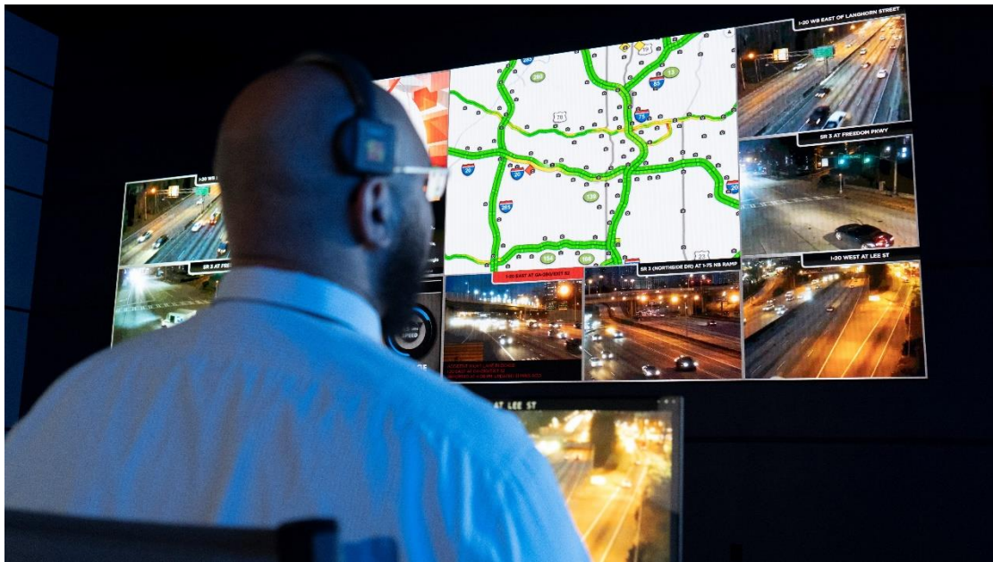
Traffic Management Center – video wall
